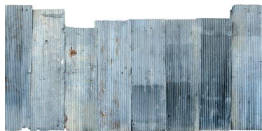
Damaged iron sheets
